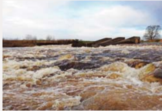
▲ Broken Scar Weir
